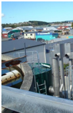
Balclutha Water Treatment Plant
