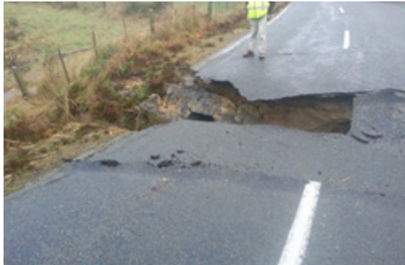
June 2015 flood-related damage to Glenledi Road
