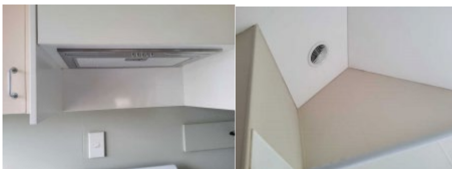
Naish Court inbuilt rangehood with new joinery and bathroom extractor fan.
