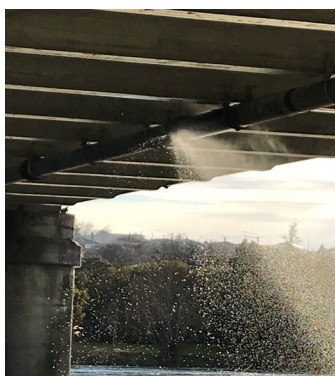
Water Leak under the Balclutha bridge
