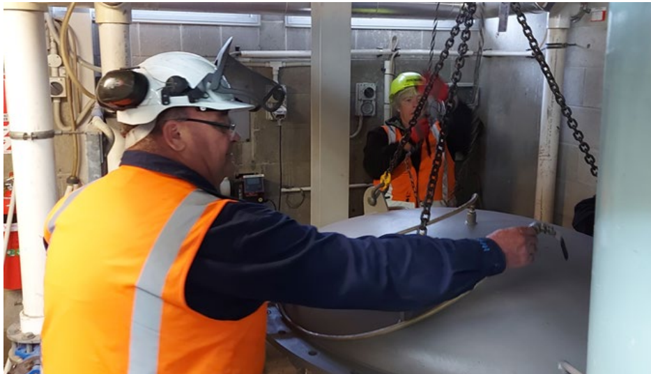
The cleaned and installed filters tubes. Ready to do their job for the next year
