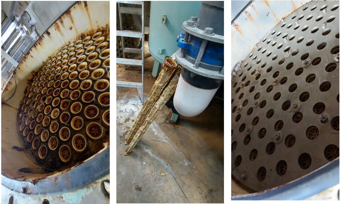
The filters to be cleaned
