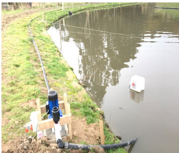
Pond Recirculation System
