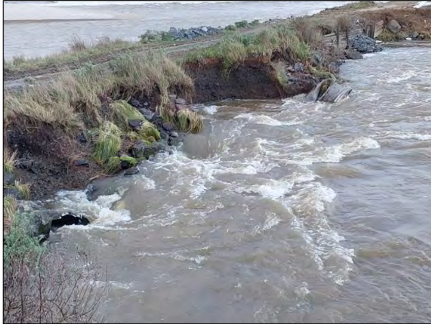
Figure 9: Erosion damages to the southern (Puerua River) side of the Koau mouth training line structure (June 2023).
