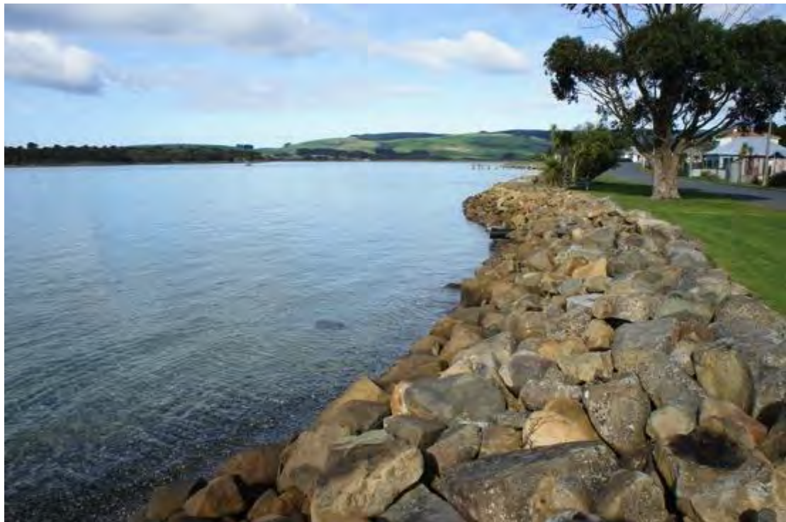
Figure 3-7 The Pounaweia sea wall (October 2019, Source: GHC).
