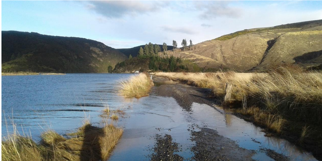
Figure 3-2 Inundation from the Taieri River onto Taieri Ferry Road. Photo taken at high tide on a sunny day (i.e., river was not in flood), June 2019 (Source: GHC).
