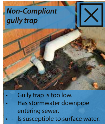
Raised off ground and covered by grate. This is an older style earthenware dish (made from clay) with the waste pipes entering the top of it.
