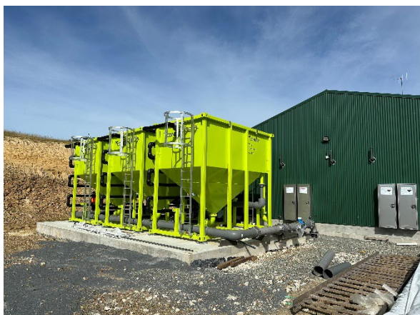
New Clarifiers and Chemical Unloading area
