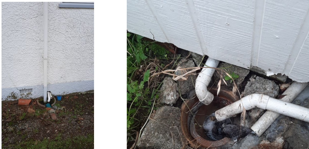
Examples of failed items in I&I inspection
