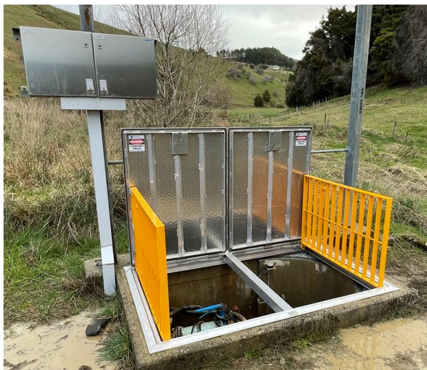
Figure 1: Puerua Water Intake - Safety Access Covers
