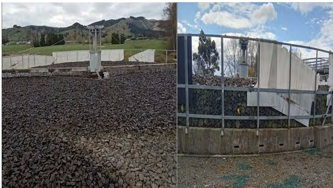
Damaged windbreak around trickling filter – Milton WwTP
