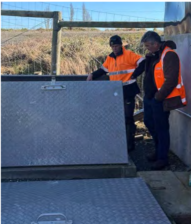
Craig Richardson (operator) & Bruce Gemmell at Stirling WwTP shown inspecting the UV filter unit
