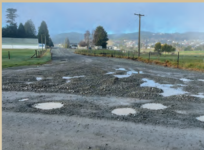
Water Street & St Albans Street pot-wholes. Credit: M. Goldsmith
