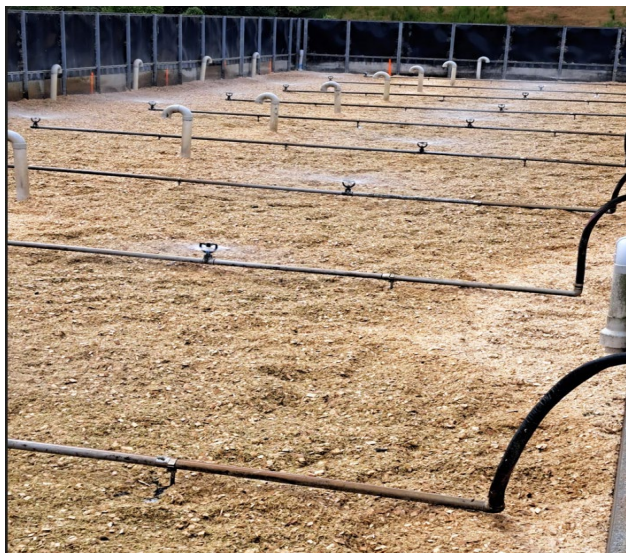
Lawrence Biofiltro bed with new woodchip February 2024
