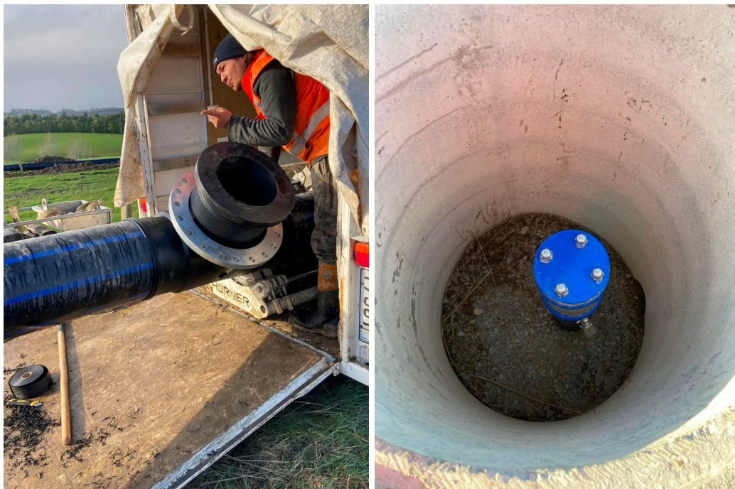
PE pipe Tee being welded and newly installed air valve in concrete chamber.
