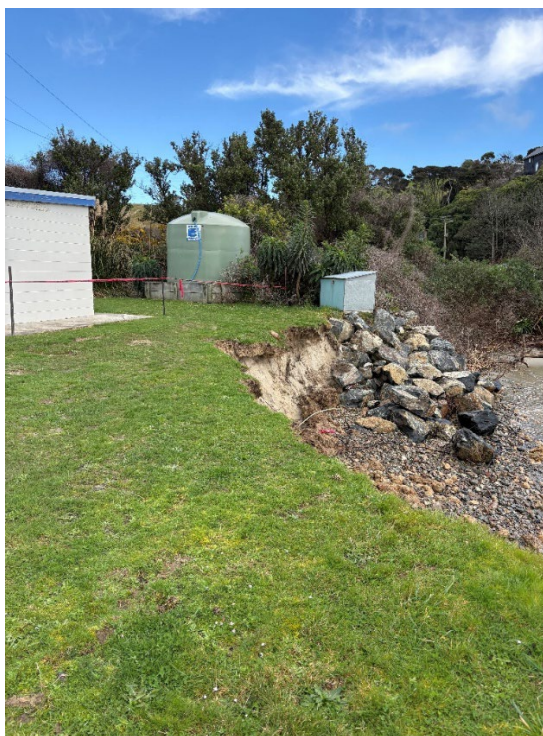
Figure 1: Knarston Park Seawall Heavily Impacted Section
