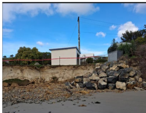
Erosion at Knarston Park
