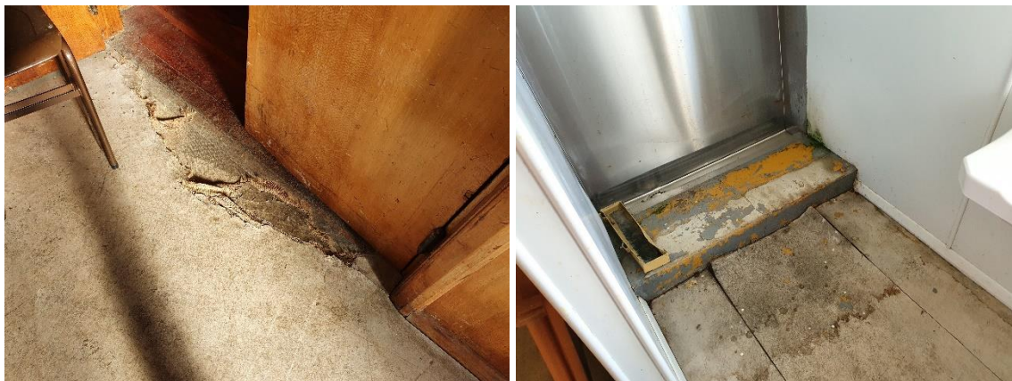
Figure 6: Damaged Lino Floor Covering in Passage (Left) & Men's Toilet (Right)
