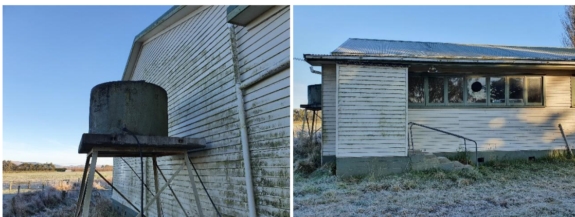
Figure 9: Unrestrained Water Tank (Left) Kitchen Steps Settled Out of Level (Right).
