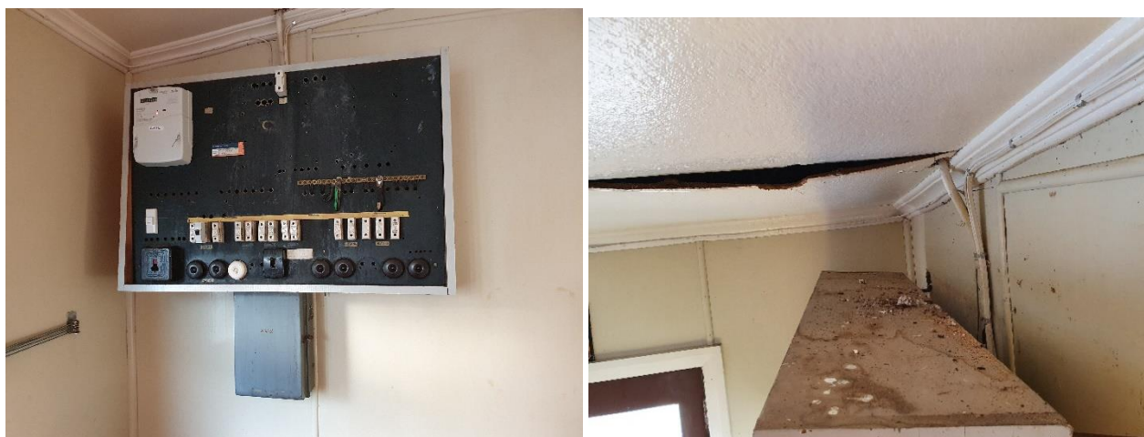
Figure 15: Main switchboard (Left) and Cabling with Rodent Damage in the Vicinity
