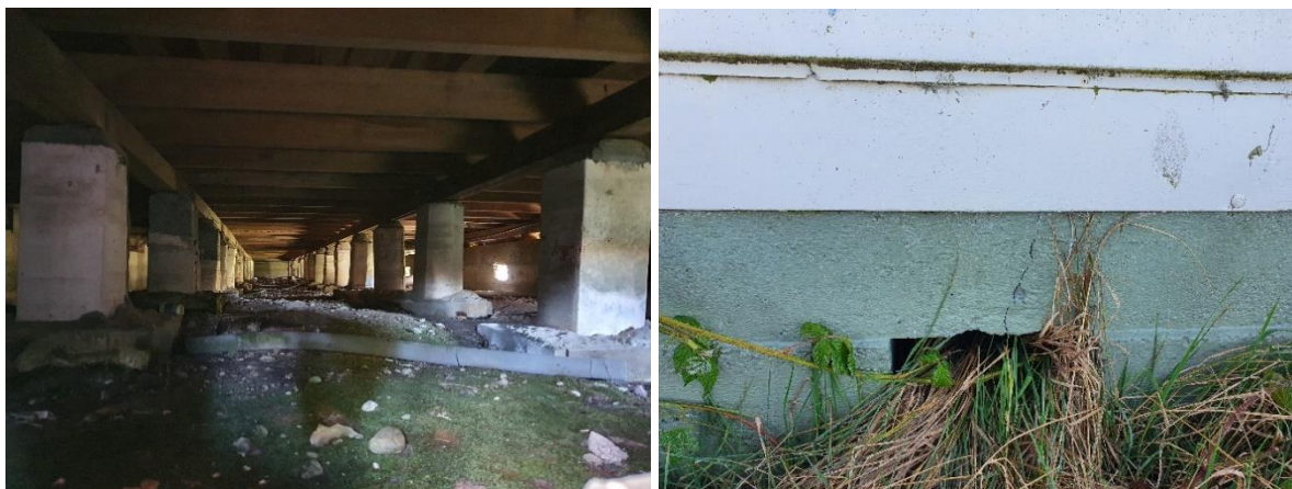
Figure 5: Raked piles under the Lean-to (Left). Typical Structural Cracking to the Perimeter Foundation (Right).
