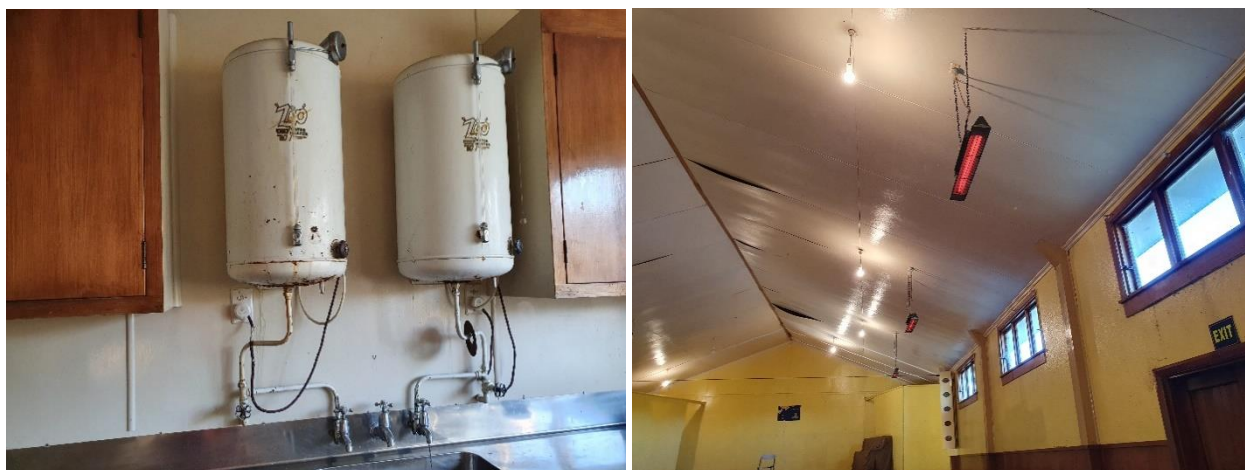
Figure 8: Twin Zip Water Heaters (Left). Hall Heaters and Lighting.
