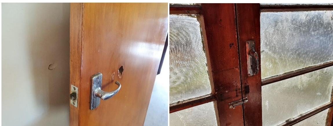
Figure 12: Minor Impact Damage to Walls and Doors (Left) and Faulty Front Door Latch (Right).
