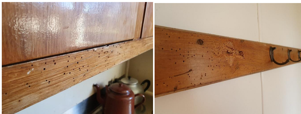
Figure 10: Borer flight holes in interior timberwork.
