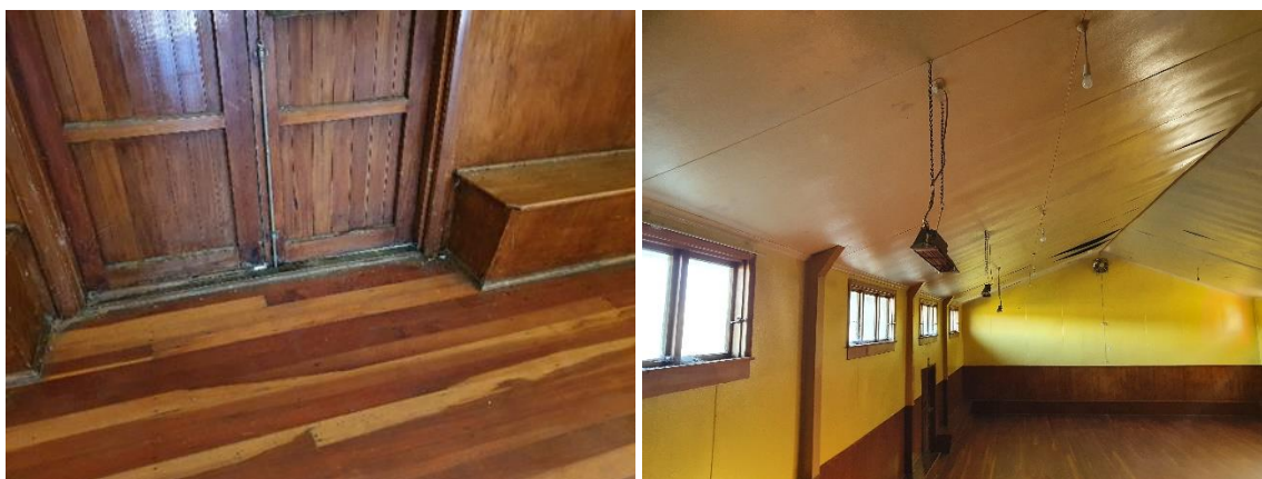
Figure 7: Broken weather strip on Exit Doors (Left). and Sagging Hall Ceiling Linings (Right).
