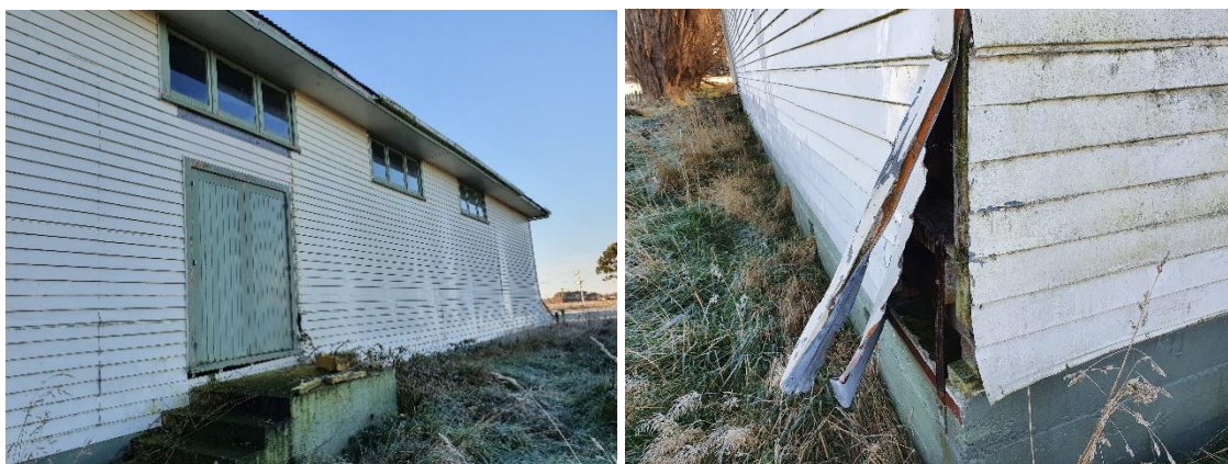
Figure 8: Collapsed Back Porch (Left). Damaged Cladding (Right).
