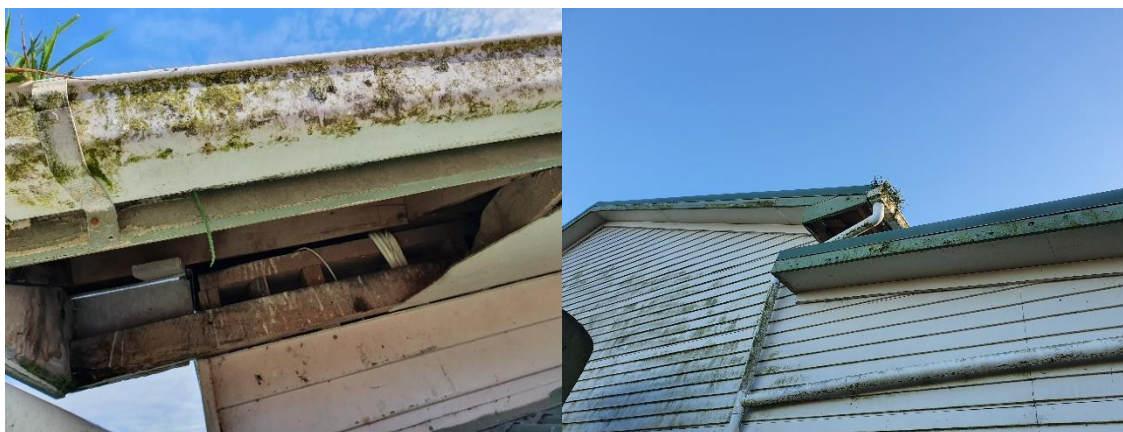
Figure 7: Damage to Soffit.
